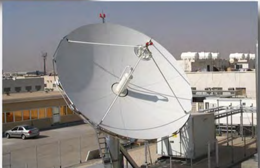
One of our Hub stations in KSA
