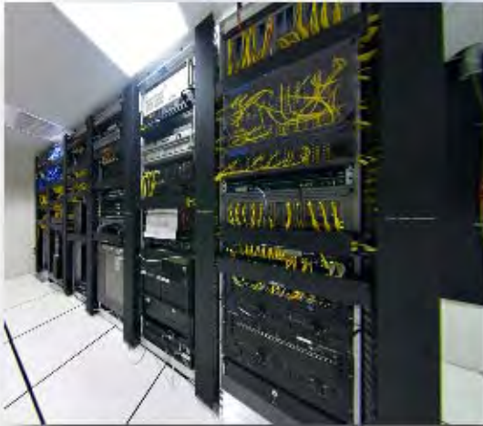
Switches, Routers and Servers
