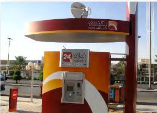
ATM machine backhauled by VSAT
