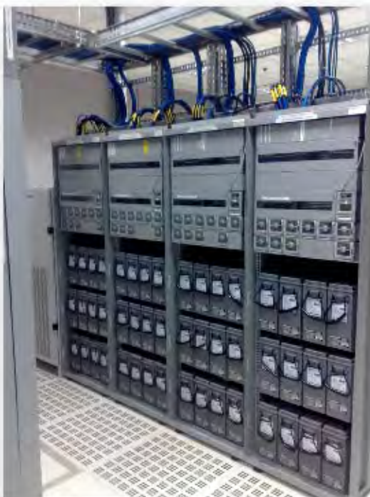
DC Power Supply System
