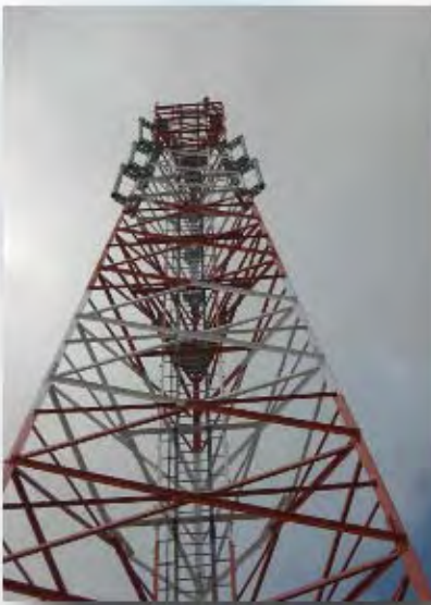
45m Lattice Tower
