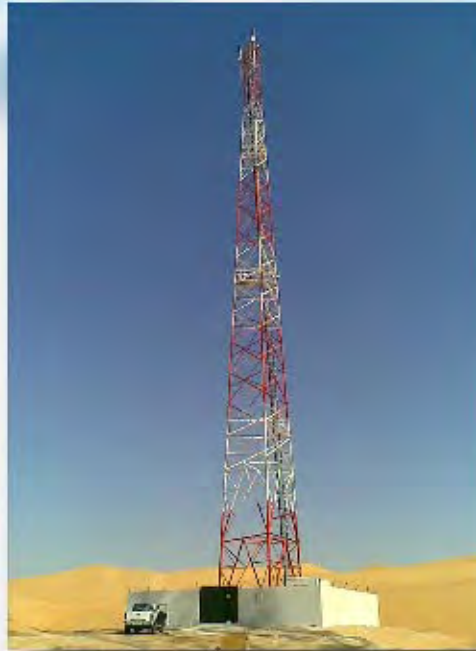
60m Lattice Tower
