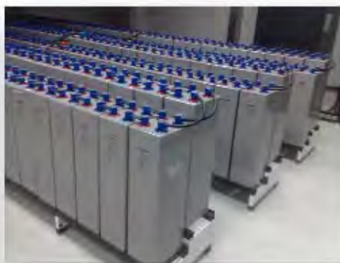
Backup Battery System
