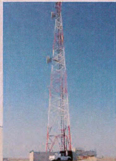
One of 32 Towers supplied and installed by Inteltec in the western region
