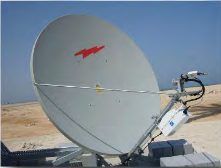
GSM Backhauling Link
