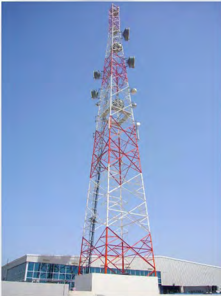
Lattice Tower 2G/3G Technology
