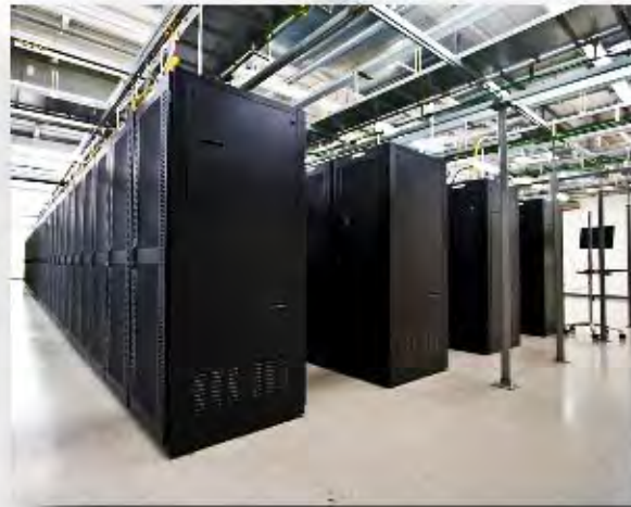
Comprehensive Datacenter Environment
