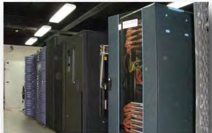
Part of our datacenter from inside
