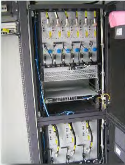
GSM Base Station
